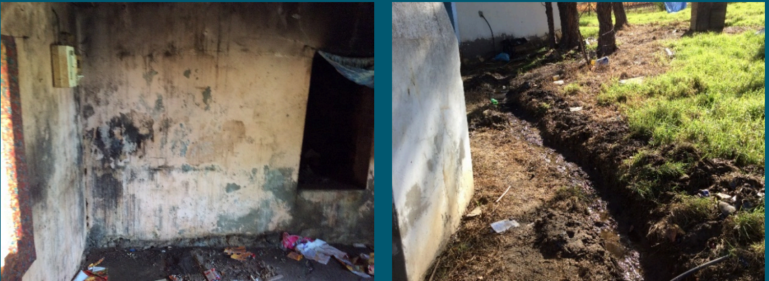
Photograph 2.3. Failure to identify a wetland seep through this area resulted in untenable damp and waterlogged conditions at this development in Sir Lowry's Pass Village.
